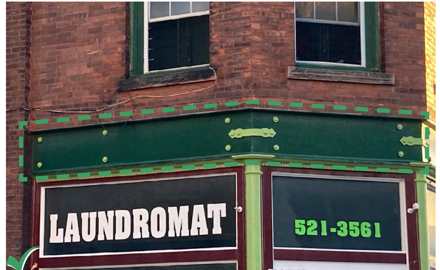
Restore and uncover steel headers. Use paint to highlight interesting details or connections.
