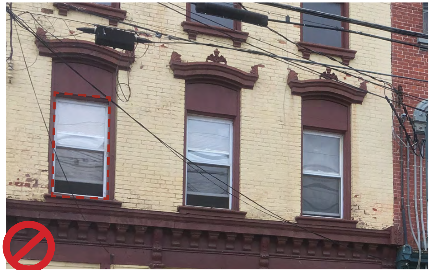
Do not replace upper floor windows with undersized vinyl replacements. Provide upper floor tenants with windows sized to the original openings.
