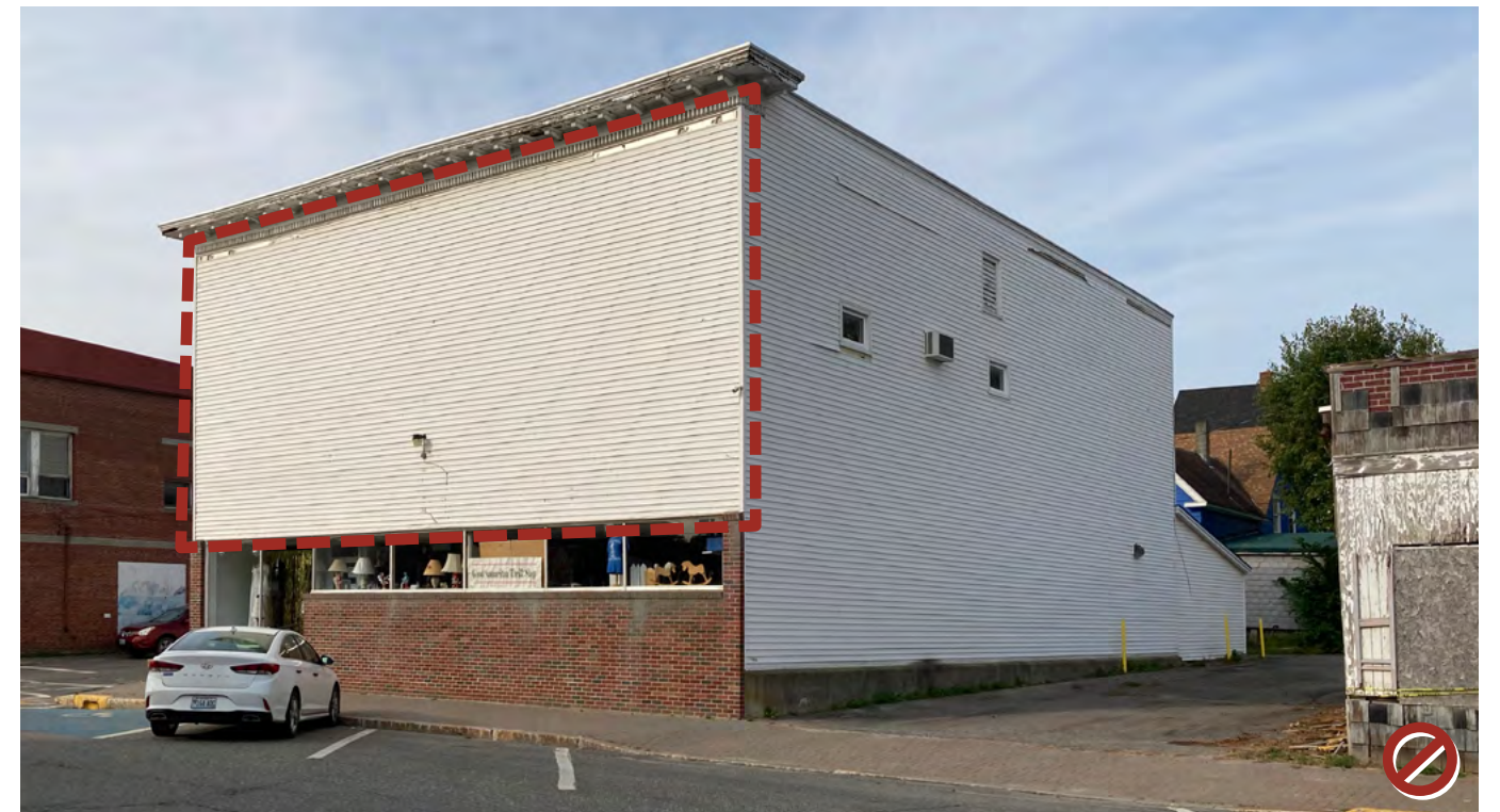
Do not cover upper floor window openings with large expanses of repetitive materials. Avoid large monotonous surfaces of just one material without articulation, depth, or color variation.
