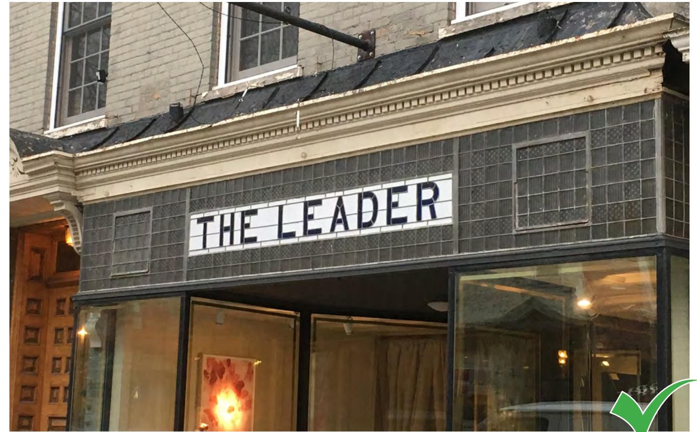
Restored transom window zones can be utilized as a unique signage opportunity.
