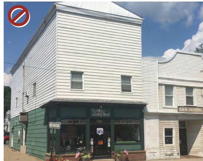
Do not use vinyl or metal siding to cover up a facade.
