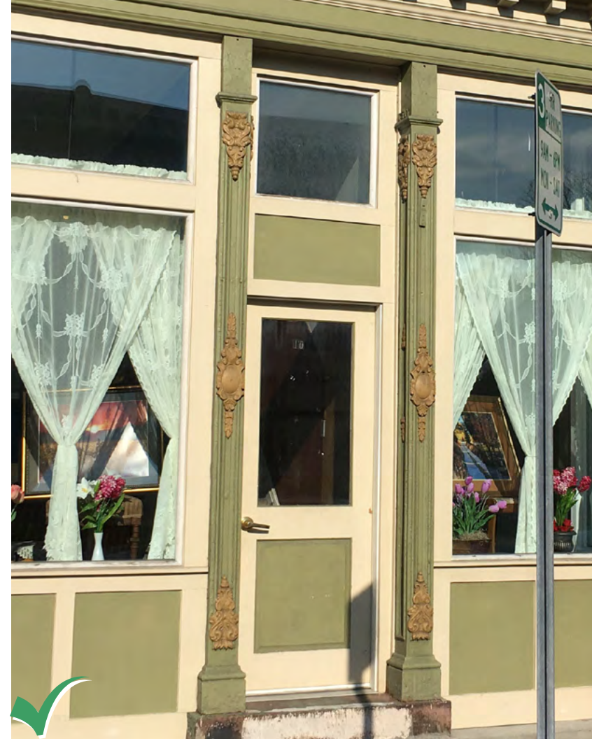
Uncover and maintain historic cast iron columns and other original facade elements.
