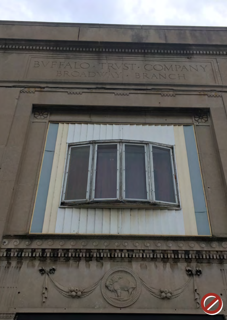
Do not fill in original openings with undersized windows, doors, or siding.
